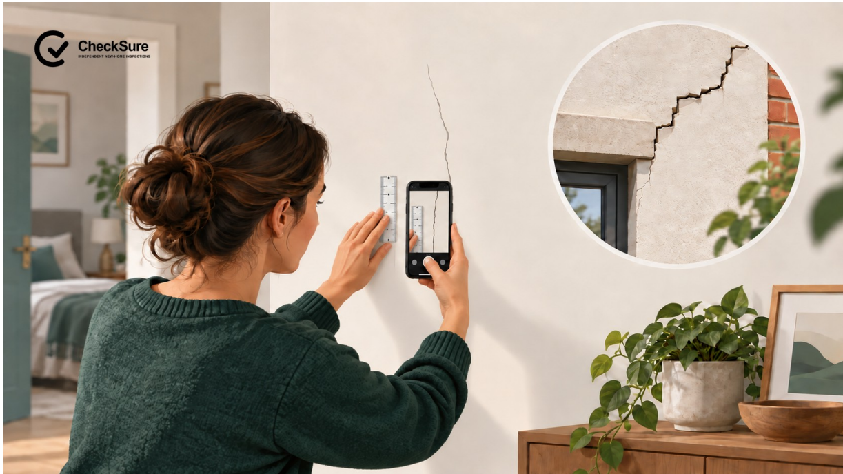
Figure 1. Record a crack with a scale and photograph so its width, pattern and change over time can be assessed.
